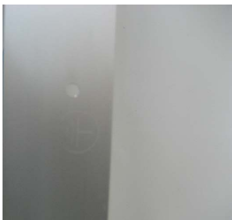
Fig. 9: Detail view of grounding mark
